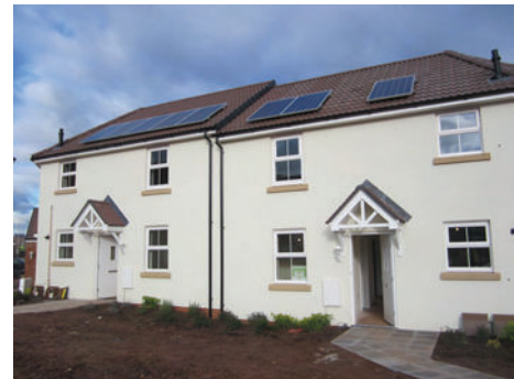
Picture 12 Photo-voltaic roof panels
